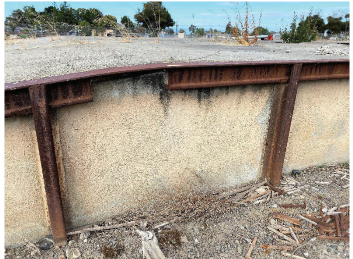
Photo 8 View southwest detailing of the concrete foundation and loading dock adjacent to inactive lines. ICF 2022.
